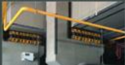
Turbine table isolation on GERB Spring elements
