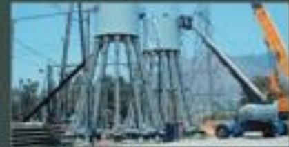
Seismic protection for substation equipment in California
