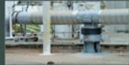
Safety related piping
