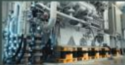
Emergency diesel generators on Spring-Viscodamper® Combination
